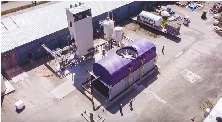
Carbon Engineering's direct air capture pilot plant in Squamish, B.C., Canada. CARBON ENGINEERING
